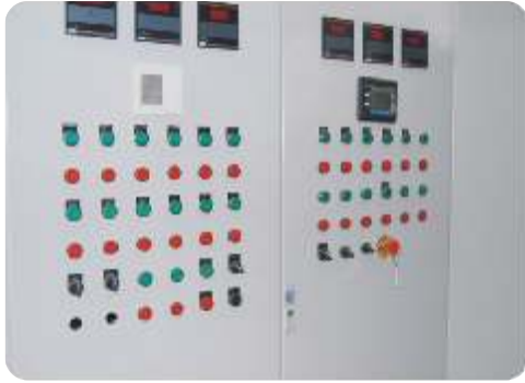
Control Panel with PLC
